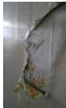
Example of oxidation after blistering
