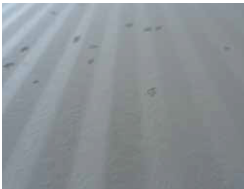
Example of blistering
